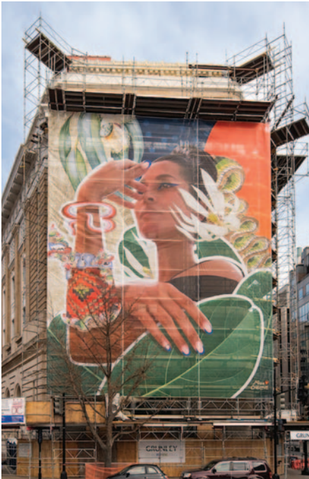
Although closed during construction, NMWA continues to engage with the public through virtual programs and dramatic displays of graphic art along the building's exterior in downtown Washington, D.C. Pictured here: MISS CHELOVE , Reseeded: A Forest Floor Flow (installation view), 2022, printed mesh 60 x 48 ft. Commissioned by the National Museum of Women in the Arts with support provided by the DC Commission on the Arts and Humanities. © 2022 MISS CHELOVE .
