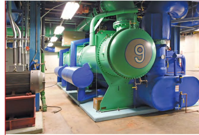
▲ 3,700-ton duplex chiller installed in 2015
