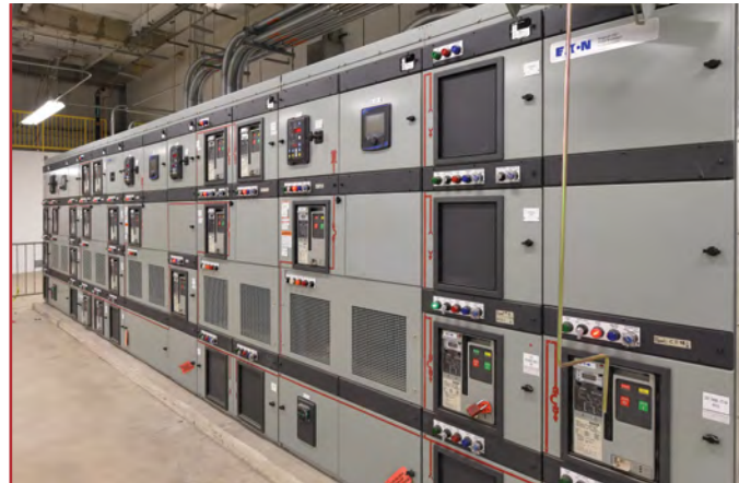
▲ 5,000-amp, 480-volt network switchgear installed in 2015
