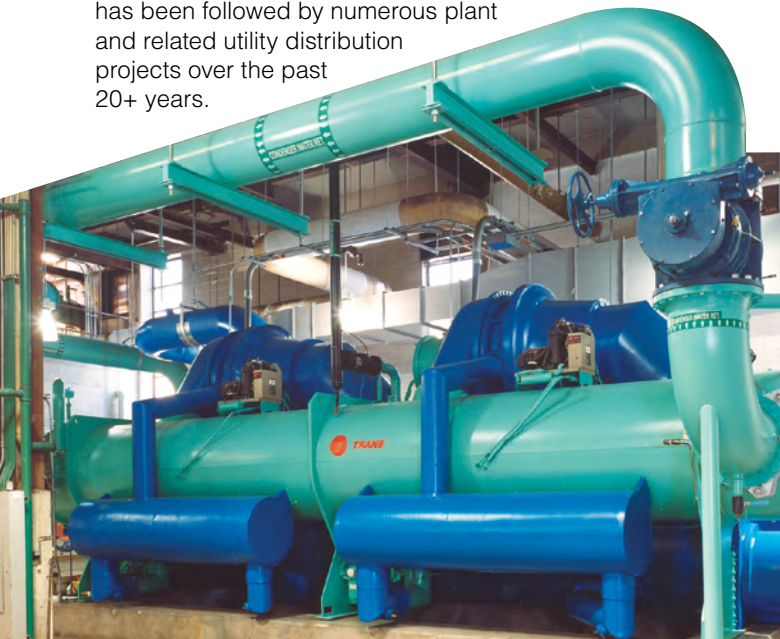
▲ 3,000-ton duplex chiller installed in 2005
