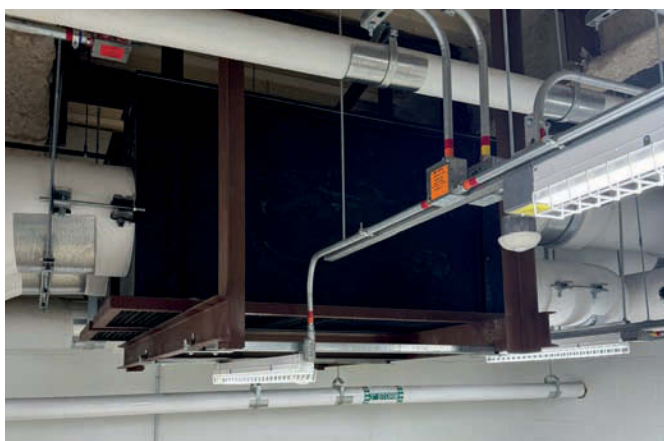
The rainwater harvesting pre-filter diverts water to the cistern for long term storage, while also diverting debris to the utility storm water system.
